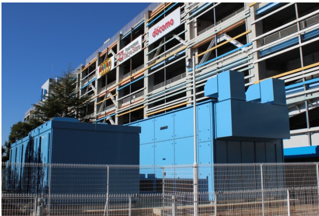
External View of the NAS battery system installed at LaLaport KASHIWANOHA
