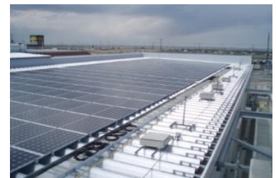
Solar power generation systems
