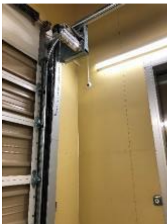
Cameras installed in the facility
