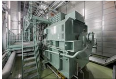
Conceptual image of gas cogeneration Japan’s first initiative to supply electricity and heat not only to areas within the development zone, but also to nearby areas with existing office buildings and retail facilities outside the project zone
