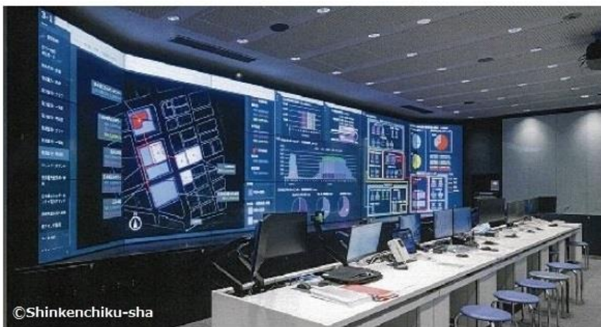
Central monitoring room
