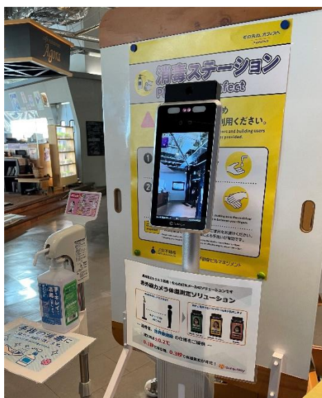
Thermocamera installed at the KOIL entrance
