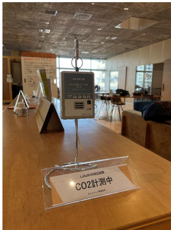
Temperature, humidity and carbon dioxide sensors installed in offices
