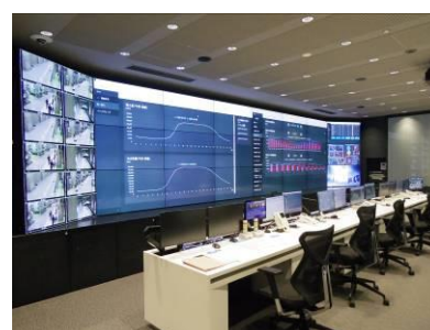
Nihonbashi Energy Center
