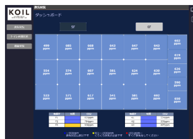
Visualization of ventilation status in an office
