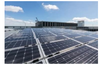
Solar power equipment (rooftop installation)
