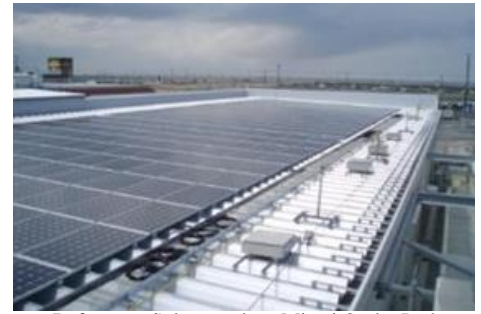
Reference: Solar panels at Mitsui Outlet Park KISARAZU
