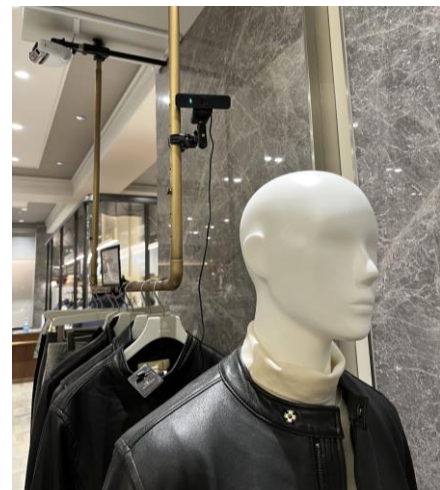
Example of AI camera installation
