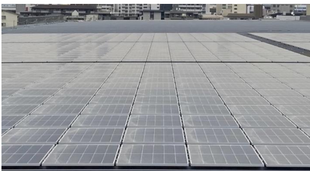
Scenes of the solar panels viewed from the rooftop Square in the Sky
