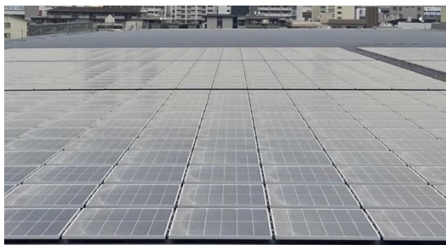
Scenes of the solar panels viewed from the rooftop Square in the Sky
