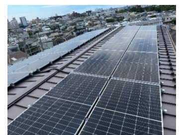
【Some of the solar panels installed on the roof】
