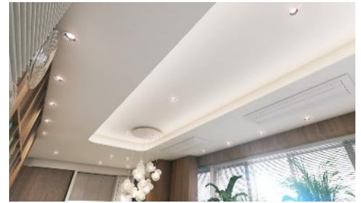
[Image of completed dimmable lighting]
