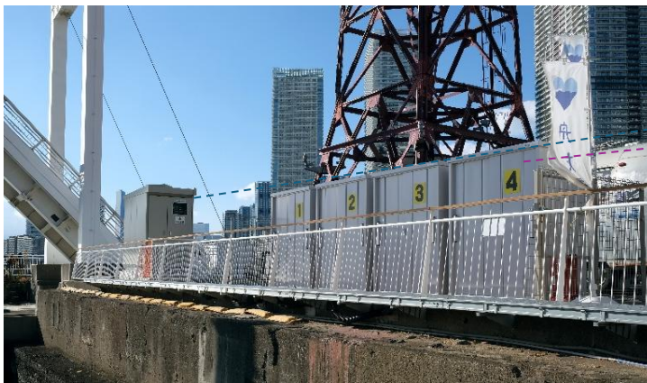
Power supply facilities adjacent to the Toyosu Pier
