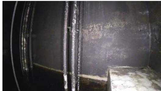
Reclaimed water treatment machine room
