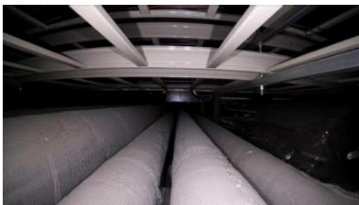
Heat source machine room
